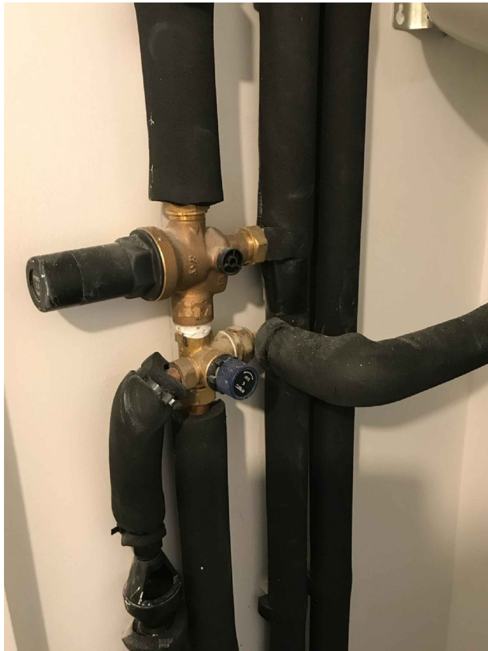
Inlet control group & Tun dish
