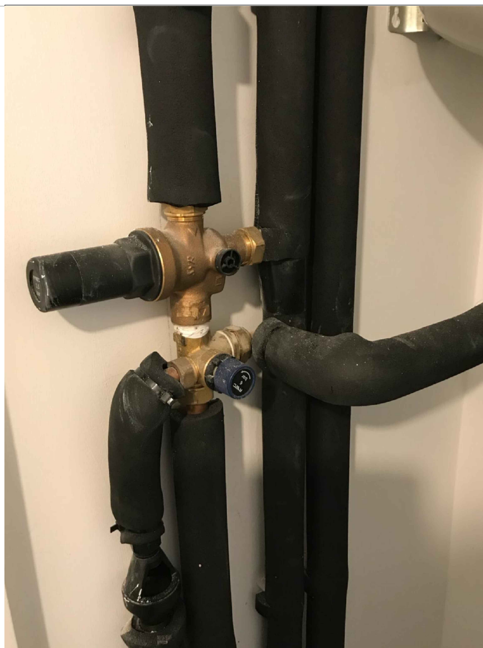
Inlet control group & Tun dish
