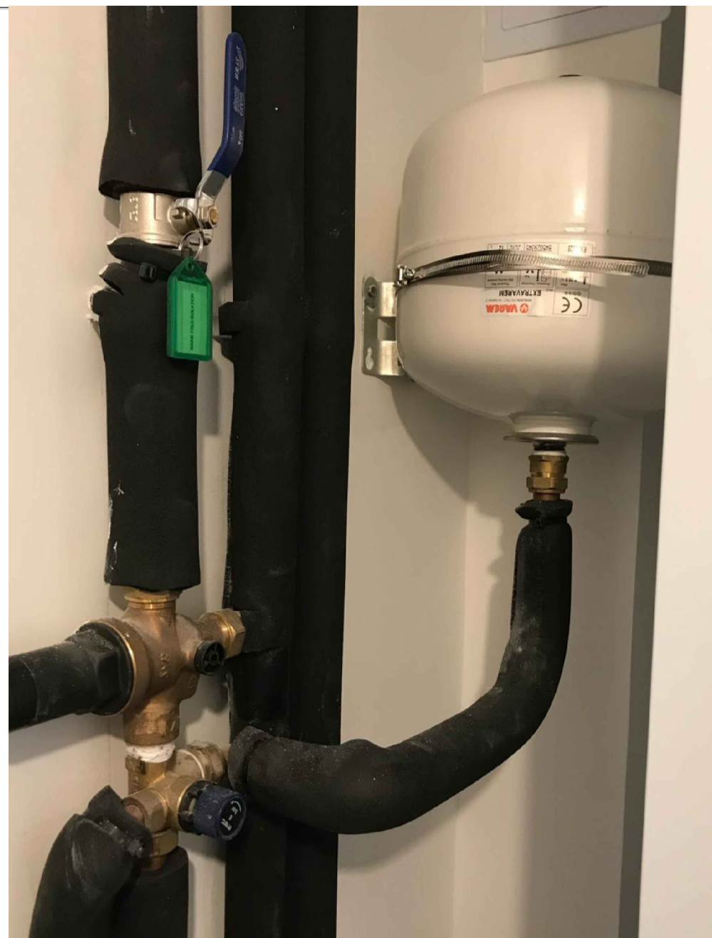
12lit Buffer vessel
