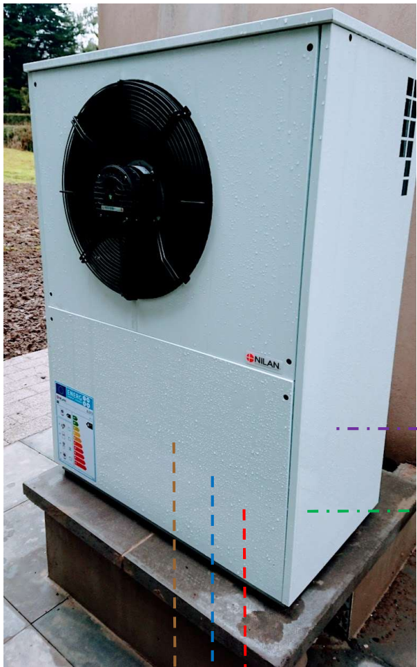
Air 9 ASHP - Outside unit
